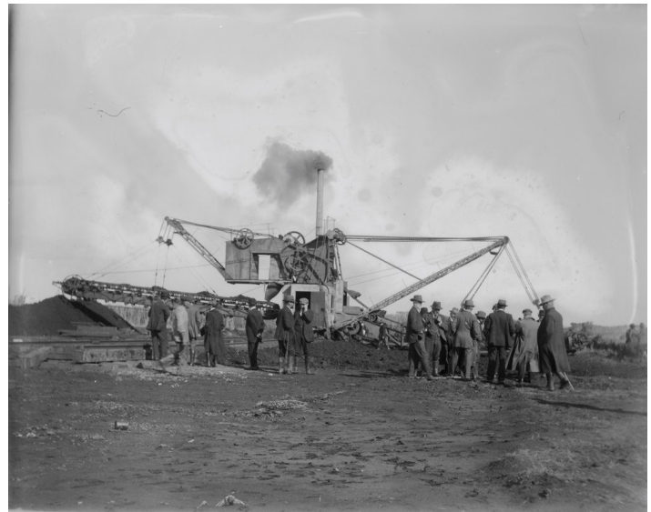
The dredge in operation on May 21, 1914, the day it was officially started
